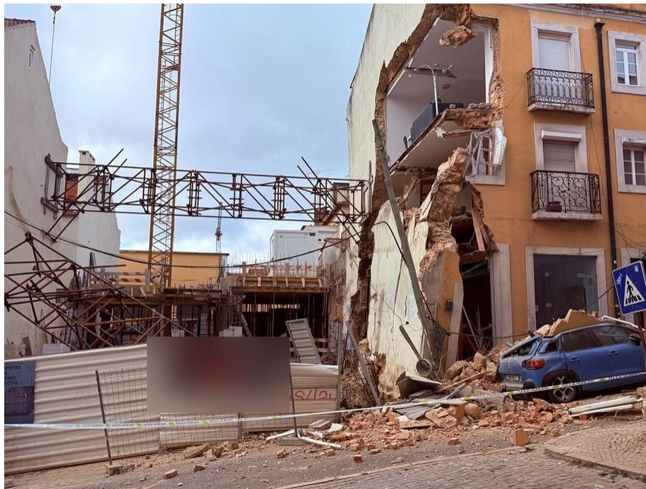
Fig. 3 — Aftermath of the incident, Rua do Sol à Graça, Lisbon, September 2025. The failure occurred on the side of the building already reliant on the support shown in Figs. 1 and 2. Site signage identifying the contractor has been redacted; responsibility for the incident remained formally undetermined at the time of writing.
