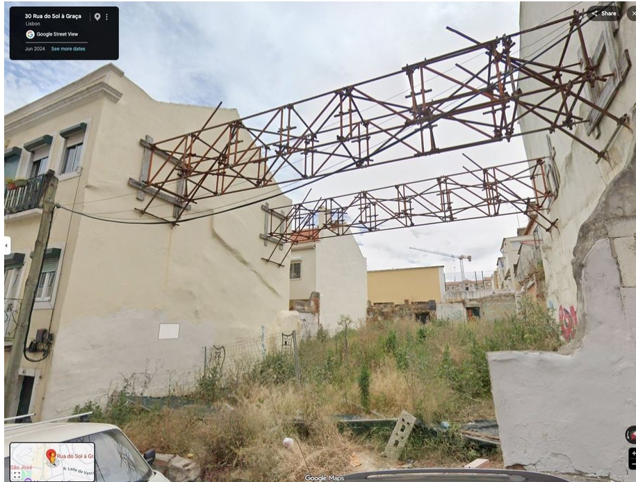
Fig. 2 — Street-level imagery, 30 Rua do Sol à Graça, Lisbon, June 2024. The same support structure remains in place a decade later, over a year before the September 2025 incident.
